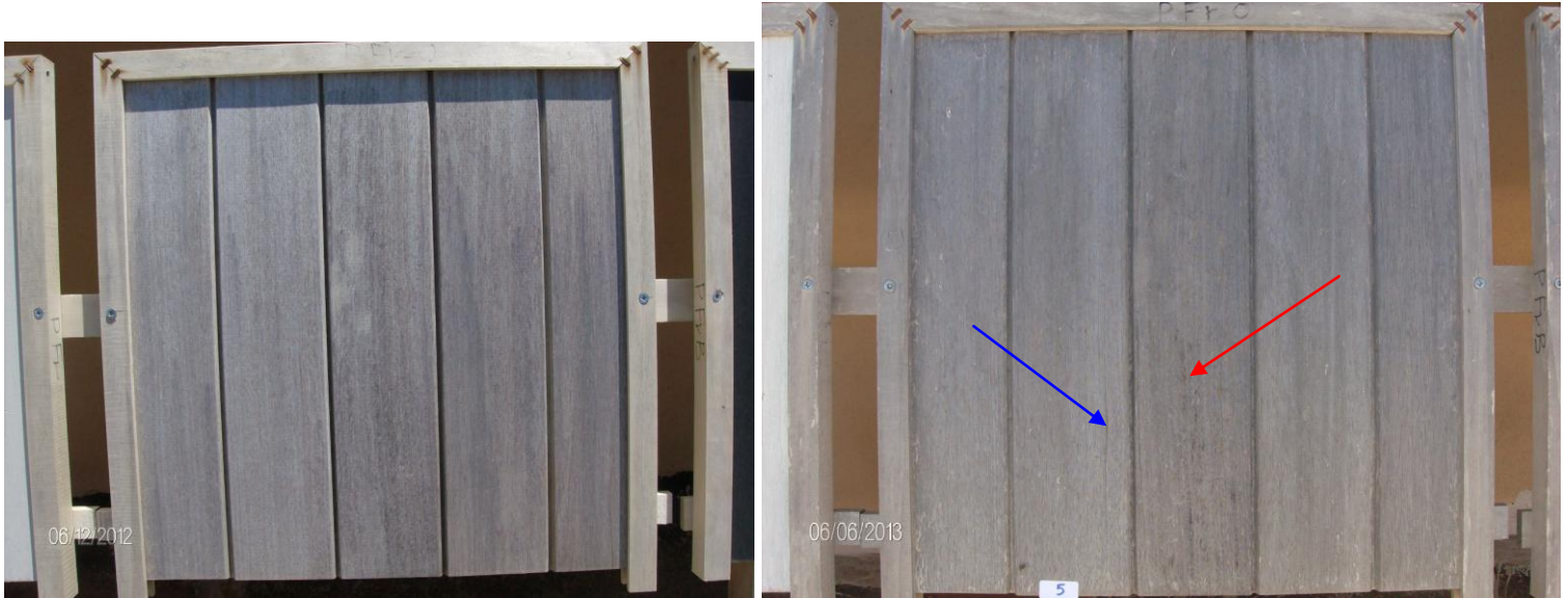
Fig. 9. Cladding 05: XXX Frake, as in June 2012; The same cladding 05 as in June 2013 .
