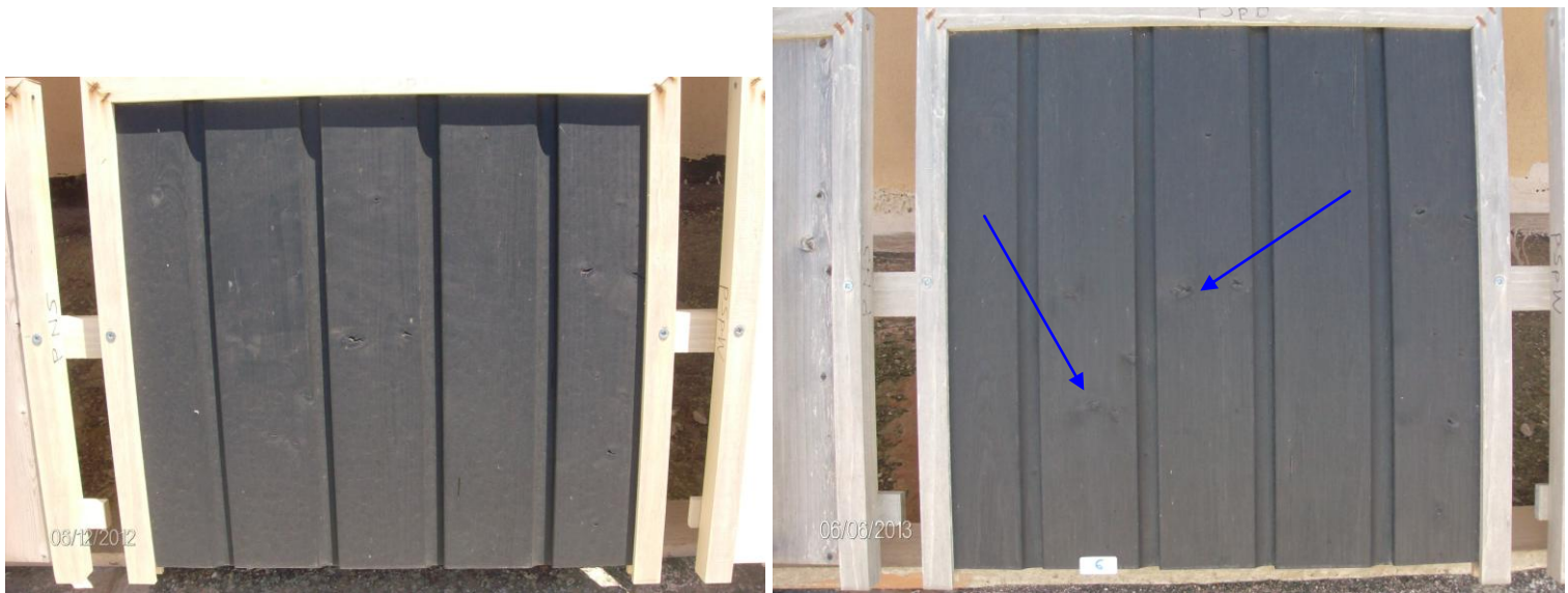
Fig. 10. Cladding 06: XXX Spruce Black, as in June 2012; (right) The same 06 as in June 2013 .
